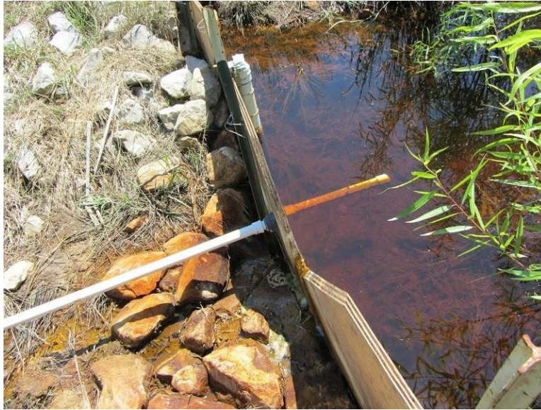
Figure 5: Photograph of weir constructed along with installed PVC to channel AMD into the test cells.
