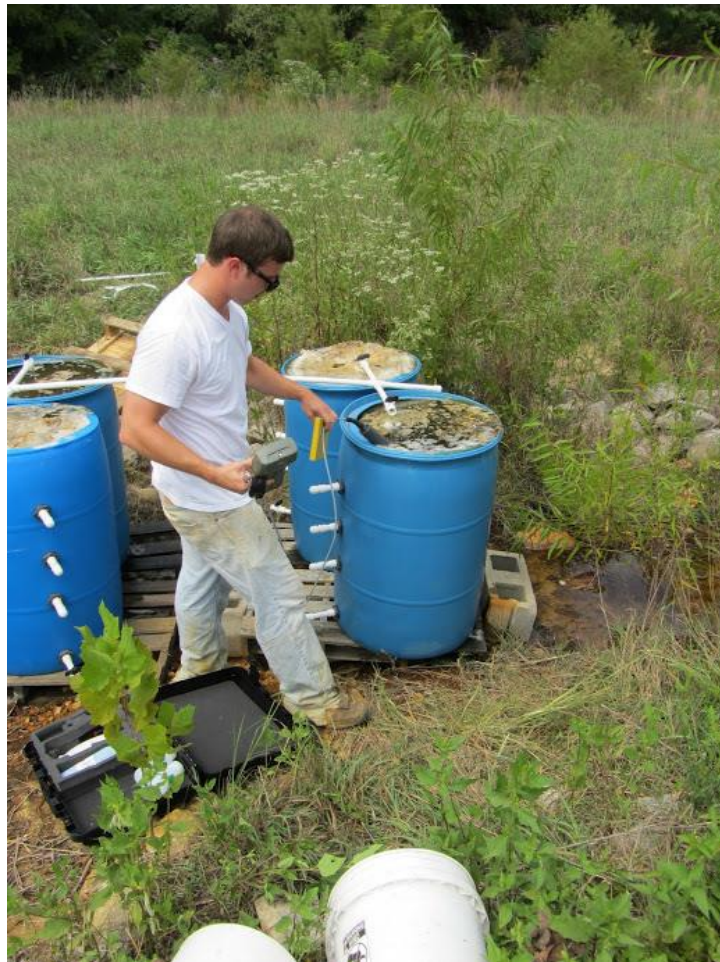
Figure 7: Photograph of reactors actively receiving AMD influent at the Tab-Simco AML site. A main PVC pipeline extends over the three pairs of reactors in which cross fittings allow AMD to be distributed in each reactor.
